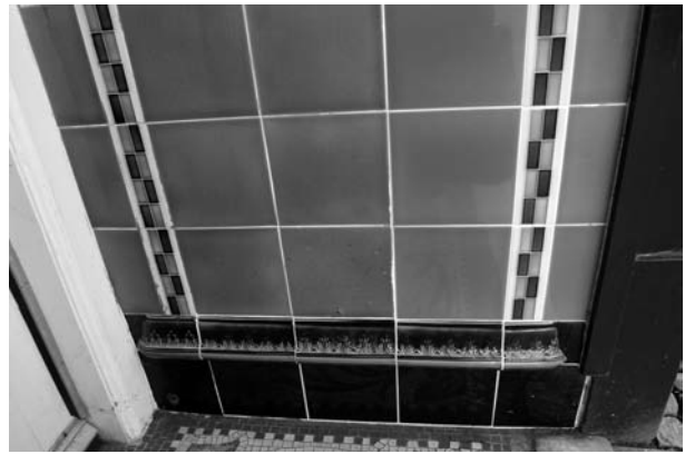
Figure 13. Lobby panel at 138 High Street, Dunbar after restoration using Craven Dunnill tiles
